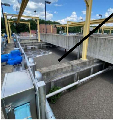
Top view of exposed Veolia MBBR system
