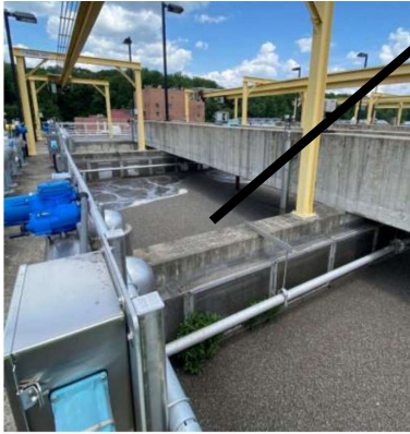
Top view of exposed Veolia MBBR system
