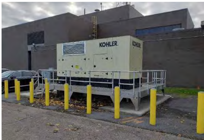
NFWB's current emergency generator is not capable of powering the entire facility.
