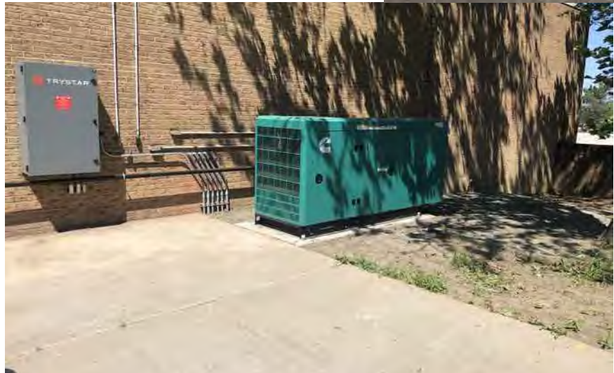
(Top Photos) New Generator at ECC North, Spring Student Center
