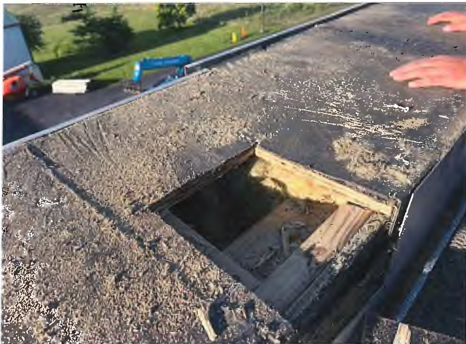
Portion of flashing and substrate was removed. Adhered directly to plywood and cannot be removed without destroying plywood substrate. EPDM flashings cannot be adhered to existing membrane.
